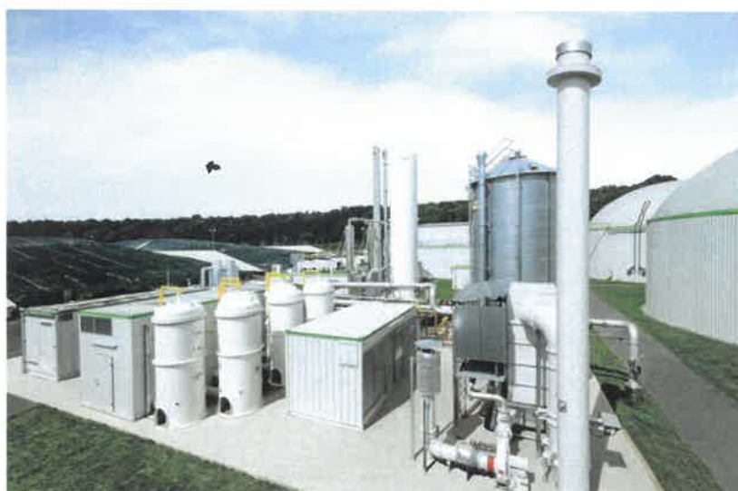
Processing plant for biomethane production installed in standard, spacesaving containers | BUP Aiterhofen
